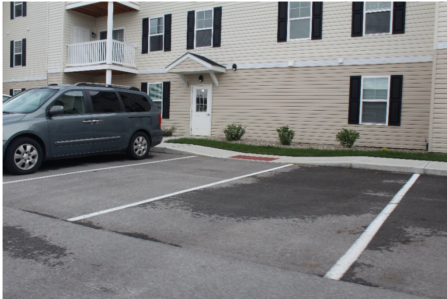
Figure E. The slopes on either side of the curb cut exceed 5% and interrupt the accessible route at Pleasant Run Senior Apartments, Indianapolis, Indiana.
