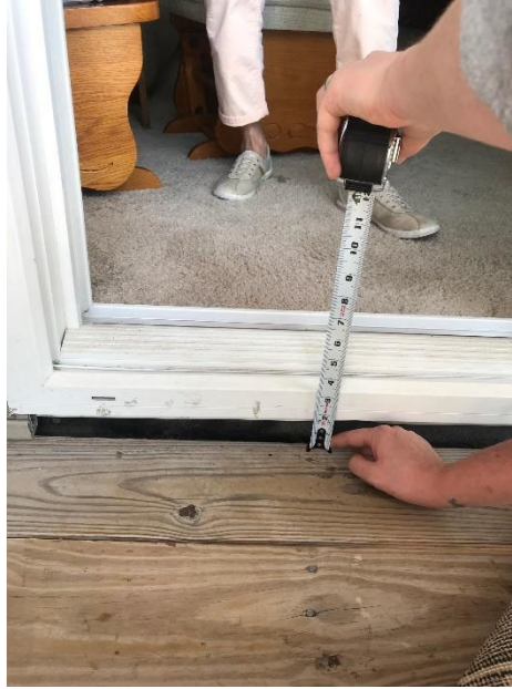
Figure G. A threshold between an apartment and a patio that exceeds \frac{3}{4} inch at Camillus Pointe Senior Apartments in Camillus, New York.
